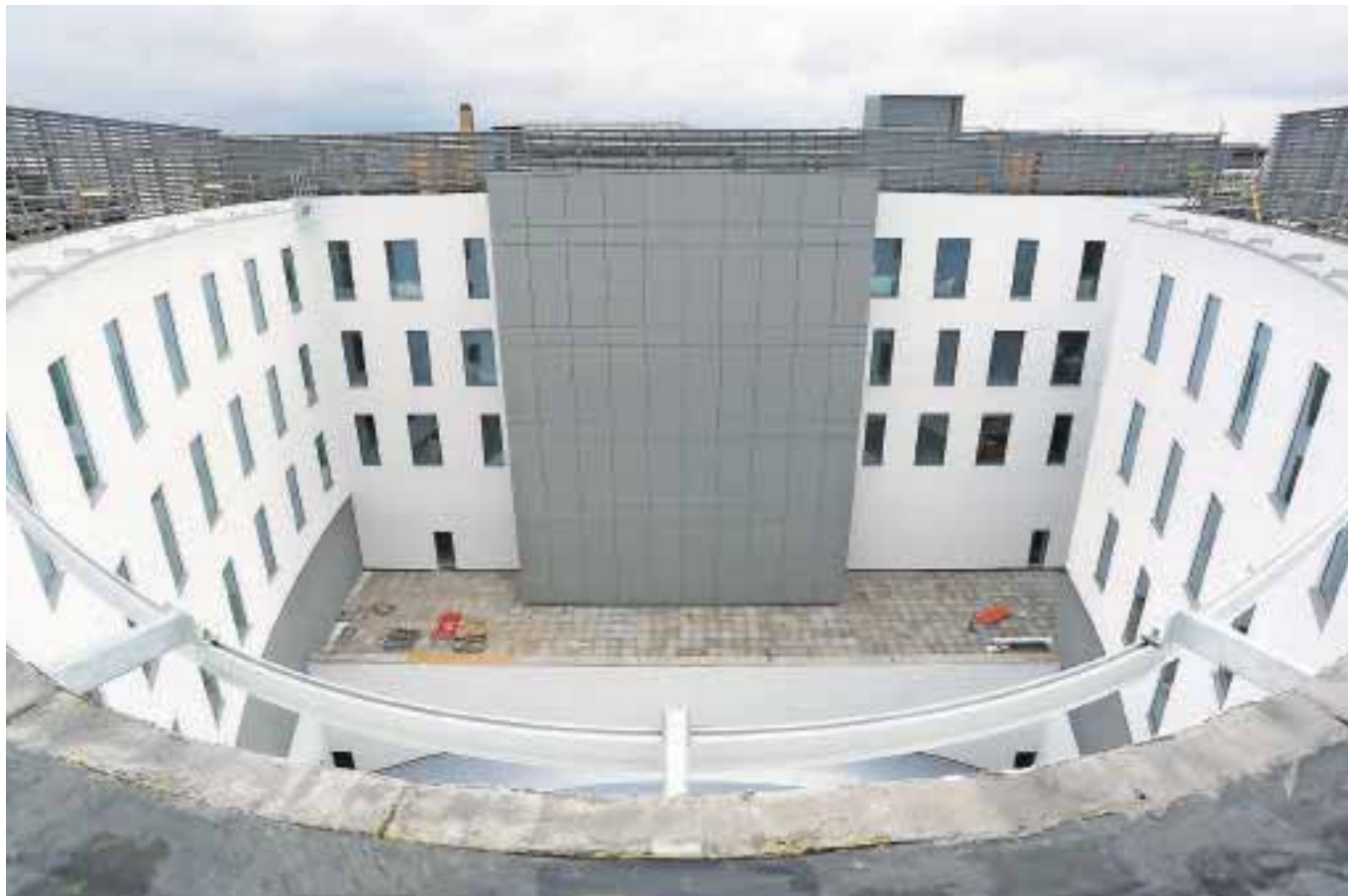
Work in progress on the Cambridge Biomedical Campus, where the world-renowned heart and lung hospital will move next year
